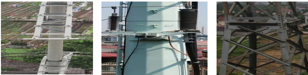
Fig. 3. High-voltage power poles
