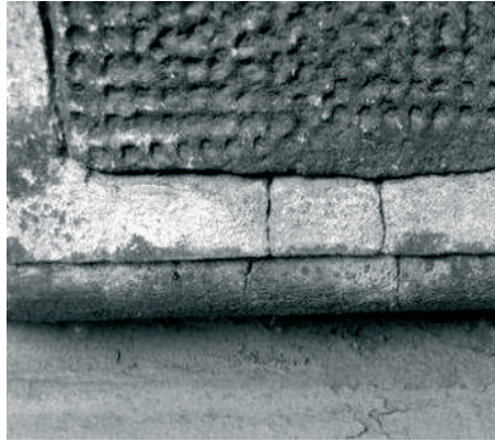
Fig. 5. The profiled pulled frame of every plank of rustication is made from Roman cement and filled inside with a help of lime plaster (on the elevation of former “Palace of Justice”). Foto M.Bevz, 2009.
