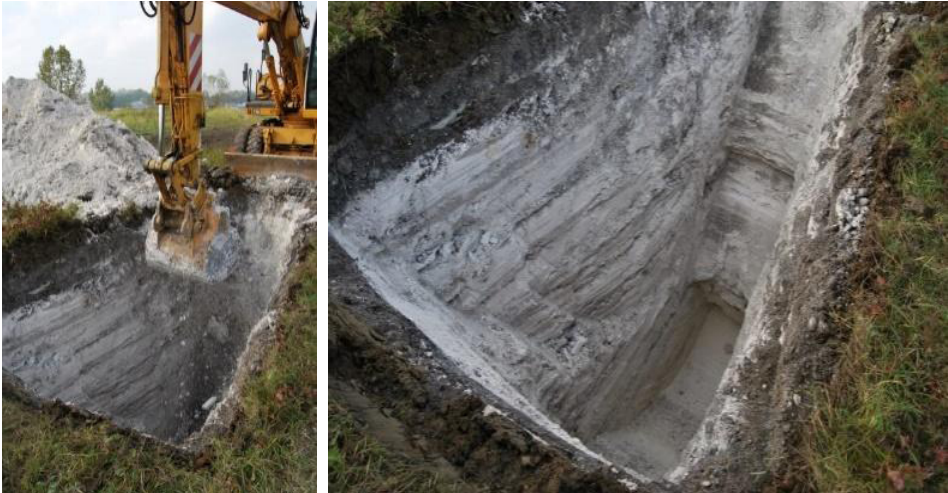
Fig. 3. The ground before starting construction works. Source: the archive of Bogumił Wrana
