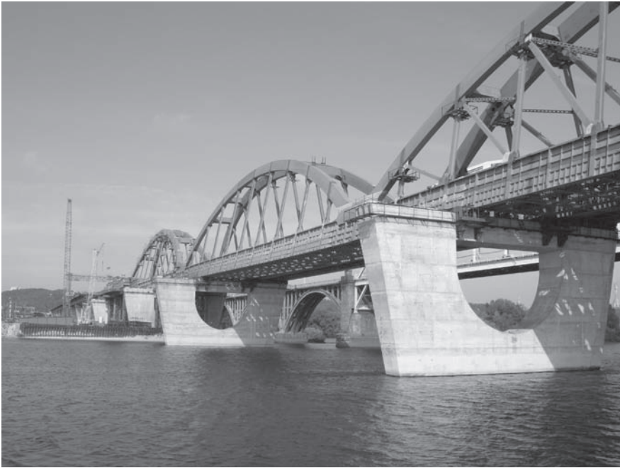
Fot. 10. Widok nowego mostu kolejowo – drogowego – Darnitski z poziomu rzeki [6]. Phot. 10. Photography of a new Darnitski railroad bridge taken from the river [6].
