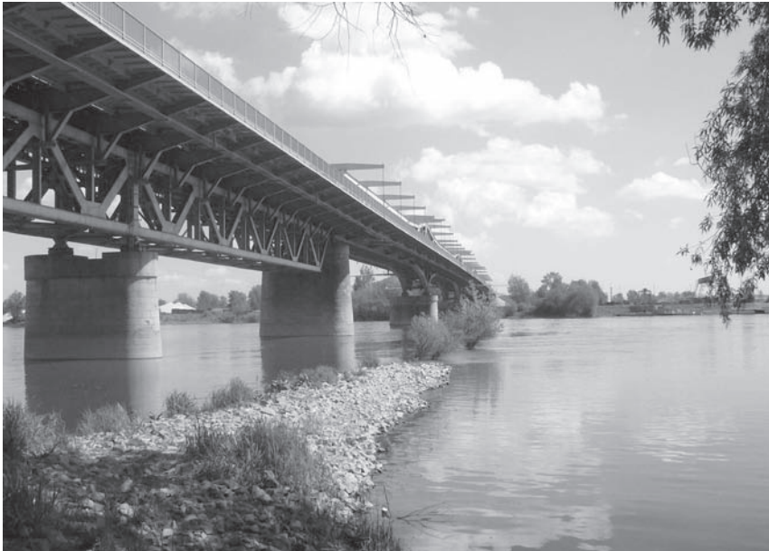
Fot. 8. Widok mostu z poziomu rzeki. Phot. 8. View of the bridge seen from the river side [6].
