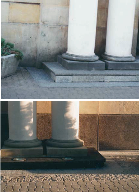
Photo 3. View of the pavement at the main entrance before and after renovation.
