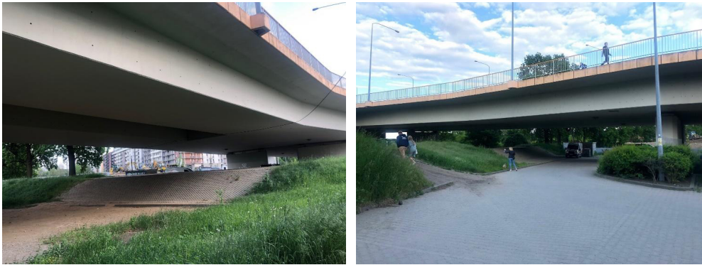
Fig. 10. Photos of the examined area. Milenijny Bridge (left-bank flyover) – crossing over the Odra River with access roads as part of the city-centre bypass, the section from Legnicka Street to Osobowicka Street, Wrocław – span № 6, between 6 th and 7 th axis – measurement axis #1. Source: author's Elżbieta Komarzyńska-Świeściak own photo archive
