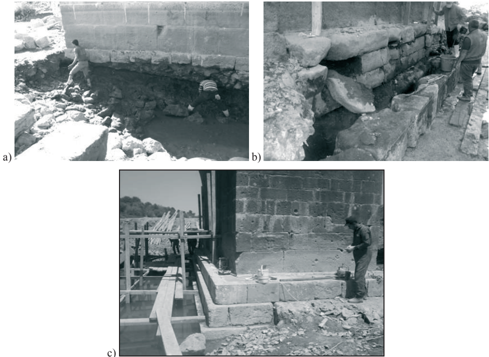
Fig. 5. Conservation works a) discharges on the grounds b-c) splits, cracks and breakages
