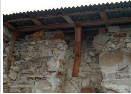
Fig. 33. Securing of the crest and a detail by a wooden construction with corrugated sheet metal (The castle in Janowiec on the Vistula River)
