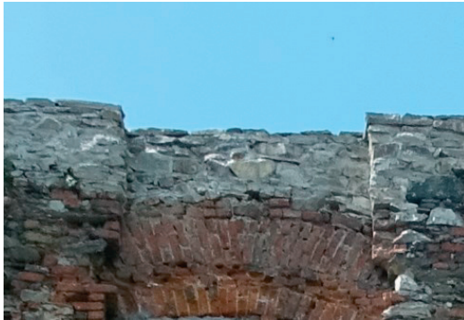
Fig. 36. Securing of the added crest with a cover (The castle in Żąbkowice Śląskie)
