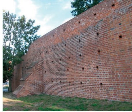
Fig. 18. Reconstruction of substantial fragments of the Wall with the material compatible with the historical one. (The castle of Łęczycza)
