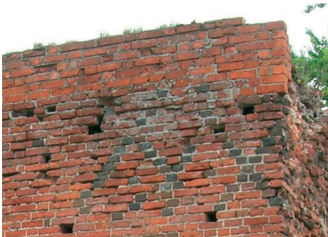
Fig. 22. Addition of the crown made of contemporary brick, on a type of mortar stronger than the original one. (The castle in Bobrowniki)
