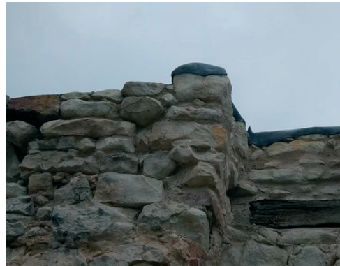
Fig. 35. The crest fragment secured with lead sheet metal. (The castle in Janowiec on the Vistula River)
