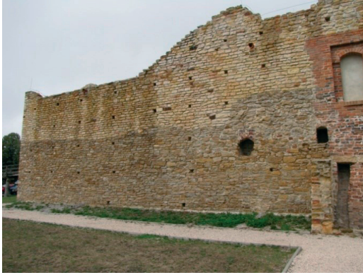
Fig. 17. Reconstruction of substantial fragments of the wall with the material compatible with the historical one. (The castle of Inowłódz)
