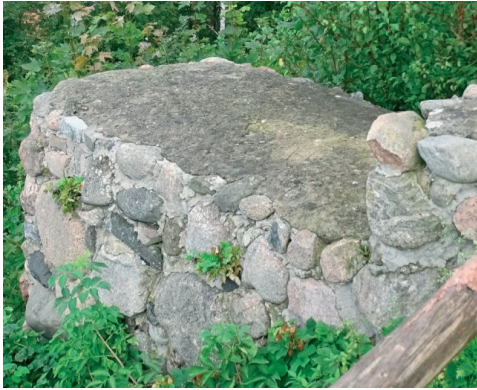
Fig. 26. The crest secured with a layer of cement mortar – with molded inclinations. (The Castle in Kurzętnik)
