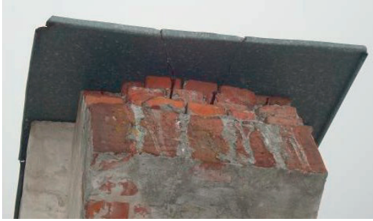
Fig. 32. A steel sheet roofing of the wall crest made directly upon the wall (The castle in Janowiec on the Vistula River)
