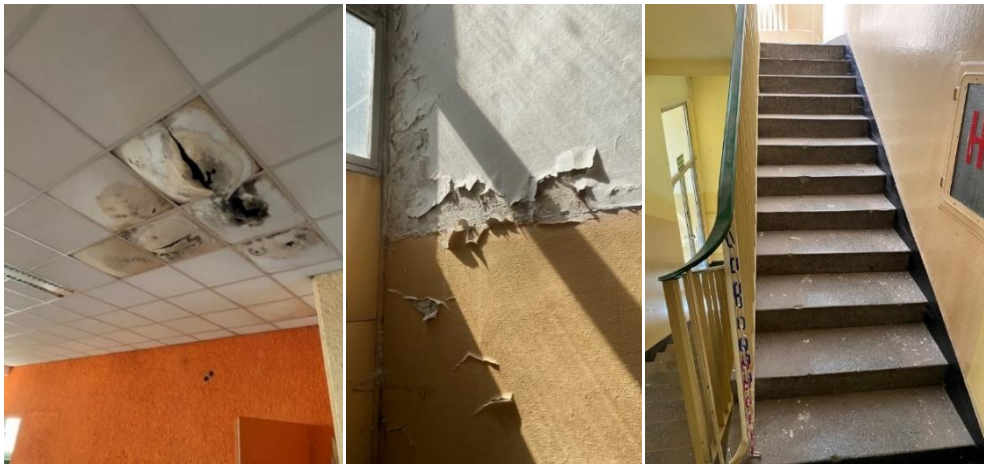
Fig. 8. Damaged cassette panels, authors' archive, 18 April 2023
