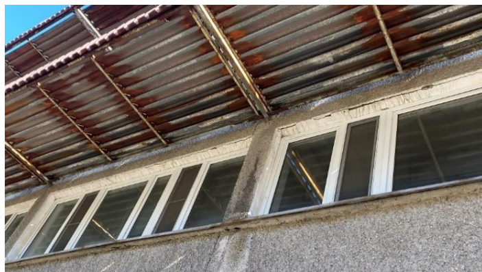
Fig. 6. Damaged elements of the southern façade, authors' archives, 18 April 2023
