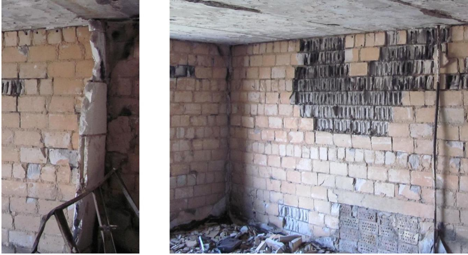
Fig. 4. The damage to the brick walls and gypsum plasterboard partitions
