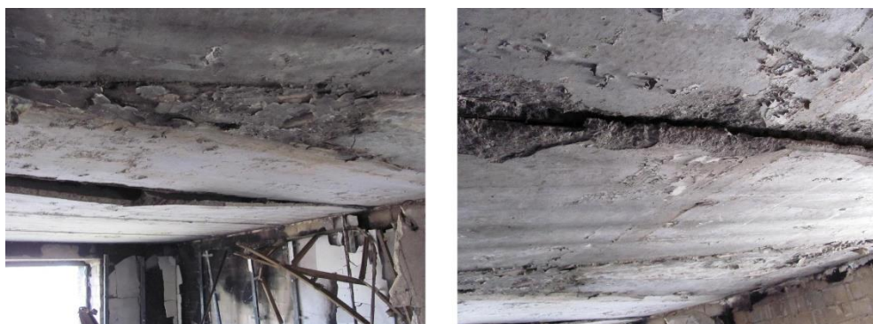
Fig. 3. The damage to the prefabricated reinforced concrete round hollow floor slabs
