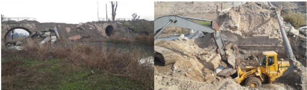
Fig. 3. The bridge before reconstruction and the beginning of rubble removal. Source: [researchers]
