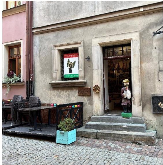
Fig. 5. Lack of handrails, damaged stairs, obstruction in the doorway, elevated outdoor seating area; Source: Author
