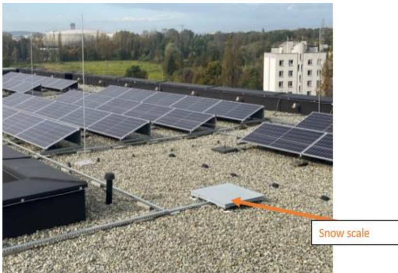
Fig. 9. Photovoltaic installation mounted on the roof (own materials)
