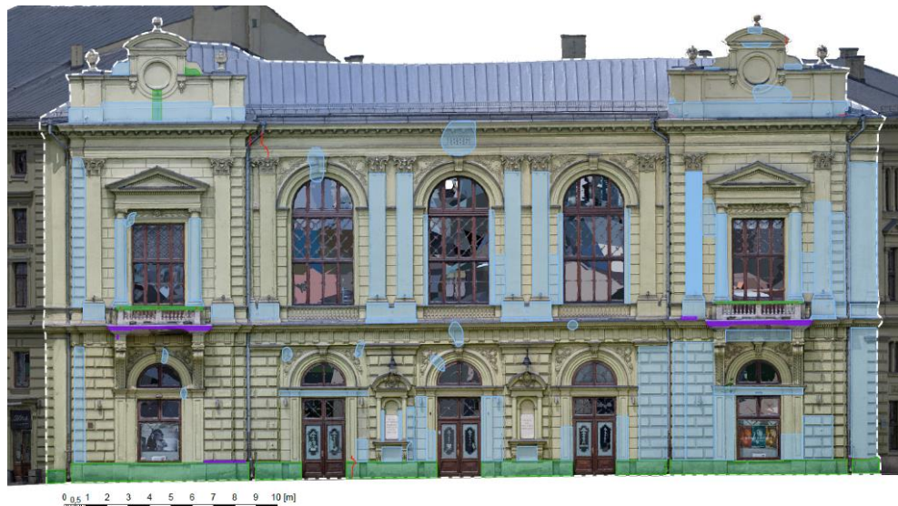
Fig. 24. Graphic inventory of the theatre façade damages
