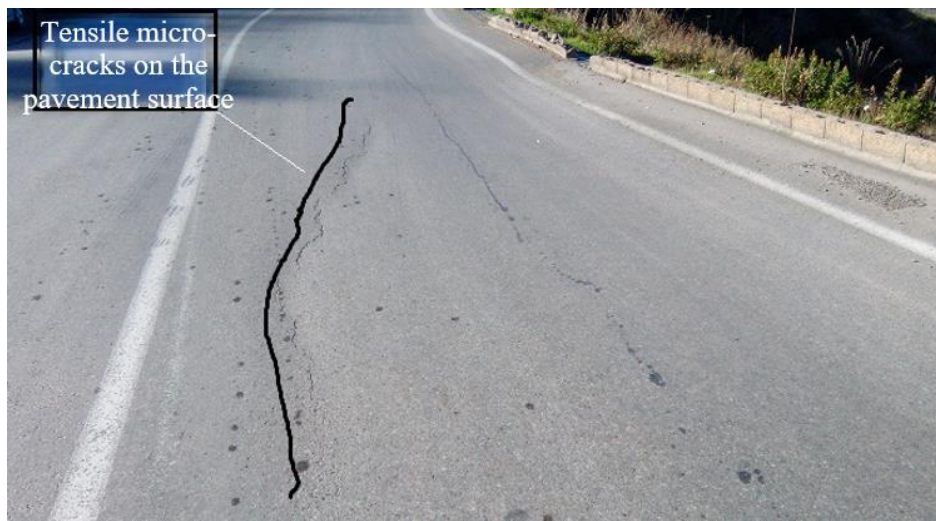
Fig. 5. Tensile microcracks along the pavement surface
