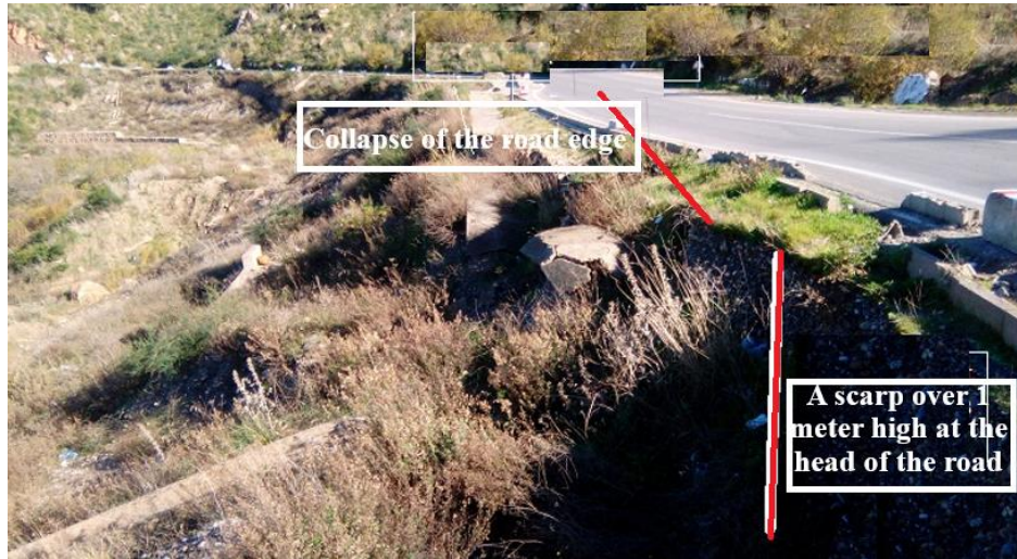
Fig. 4. Shoulder collapse and embankment failure along the roadway
