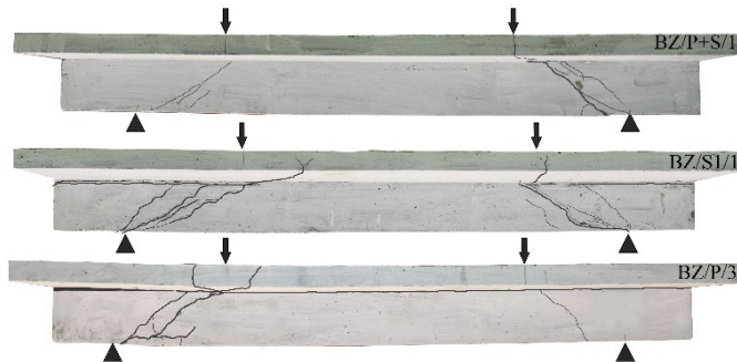
Fig. 3. Crack pattern of representative beams of the BZ/P+S, BZ/S1, and BZ/P series after failure. Source: own study
