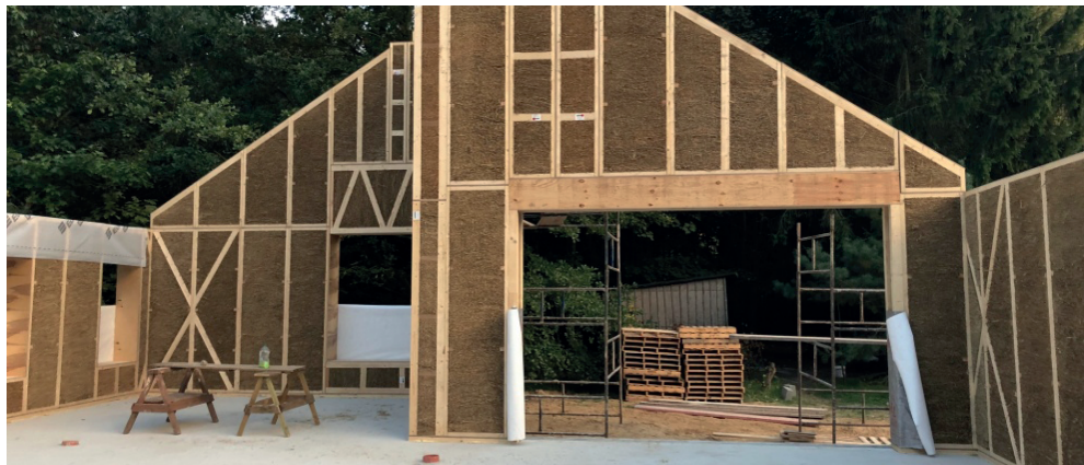
Fig. 2. Implementation of the 'ASZ Dom' project using prefabricated EcoCocon panels, Koziej Architekci office, source: www.koziejarchitekci.com [14]
