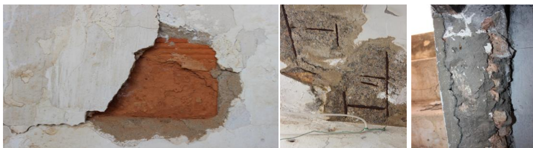
Fig. 12. Incompatible materials used to patch cracks and other defects in the mosque, source: the authors, 2018
