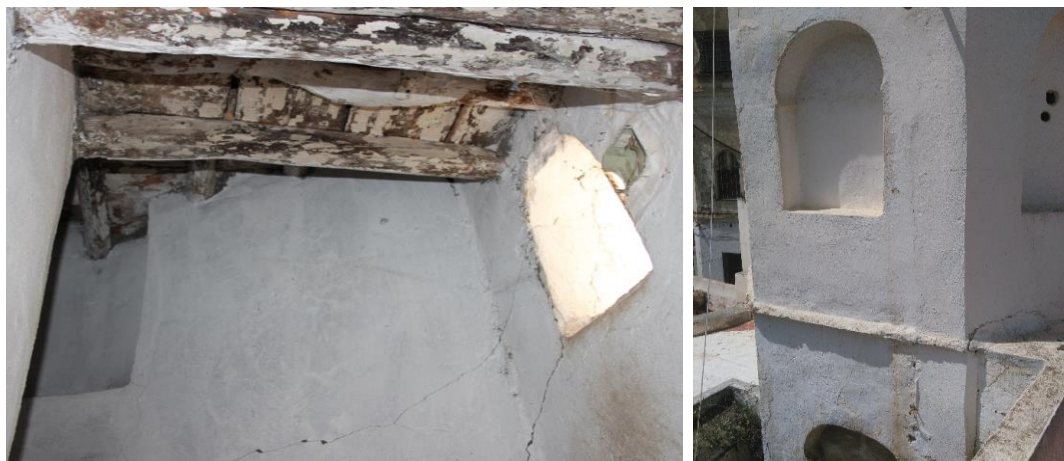
Fig. 11. Cracks recorded on the exterior and interior of the minaret, source: the authors, 2018
