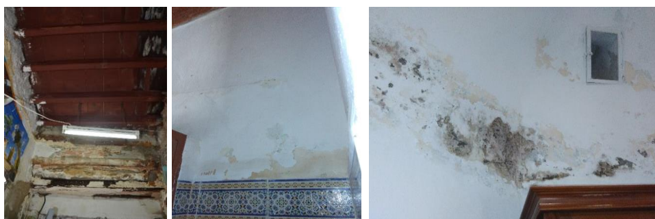
Fig. 8. Moisture-related deterioration inside the building (plaster removed), source: the authors, 2018
