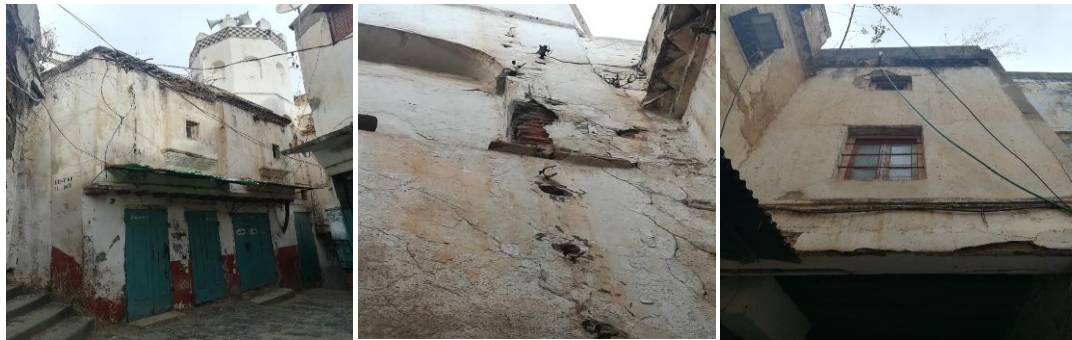
Fig. 10. Cracks and structural damage observed on the exterior of the mosque, on the minaret and prayer hall sides, source: the authors, 2018
