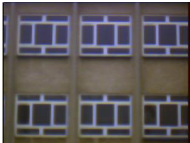
Fig. 1. A fragment of a wall of a thermal upgrading building (before thermal upgrading)
