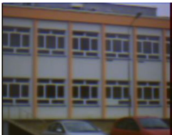
Fig. 2. A fragment of a wall of a thermal upgrading building (after thermal upgrading)
