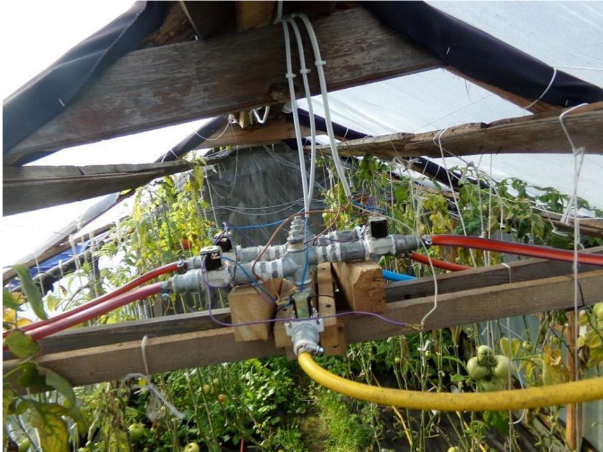
Figure 4. Connection of valves to the manifold
