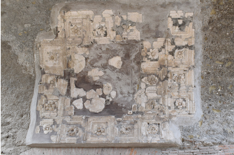
Fig. 4 Stucco Fragments repositioned on the barrel vault's inner surface on Maiuri's project. (Photo Credit: ISCR-Matera students)
