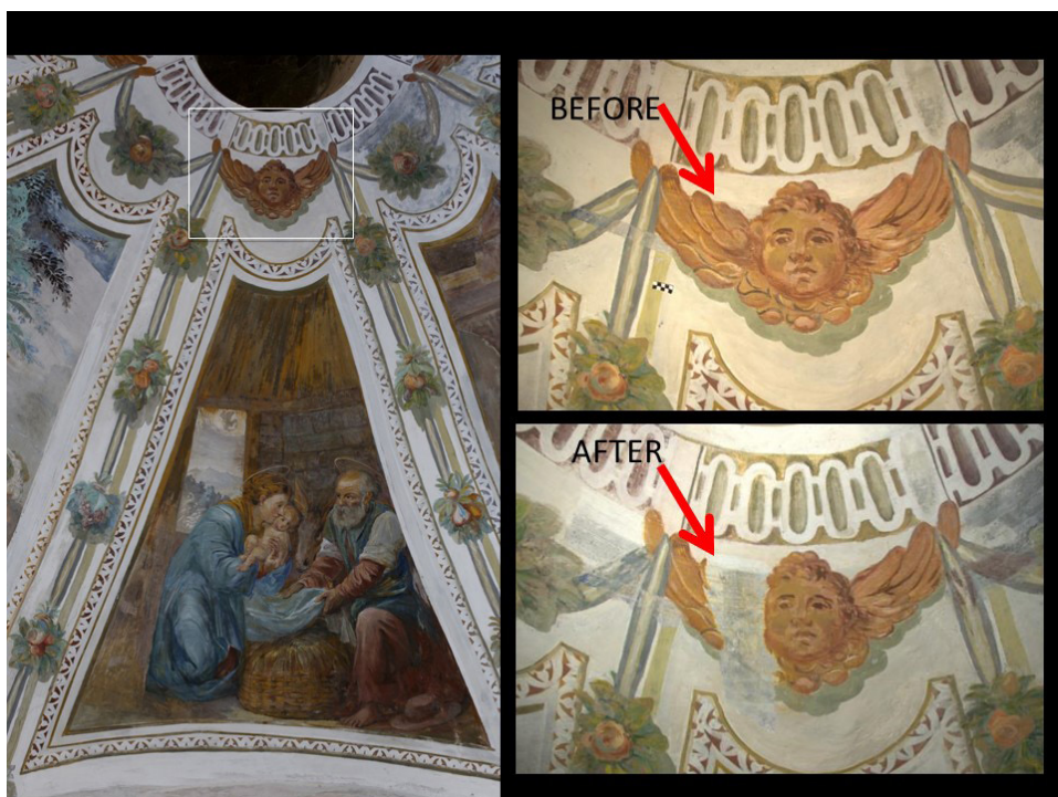
Fig. 6 Overpainting removal test in the architectural portion on the vault. The test revealed that no original paint was present underneath
