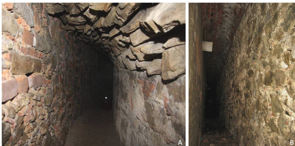
Fig. 8 Silver Mountain Fortress, insulation and ventilation corridors. A - a corridor with a 'drip' vault. (Photo: G. Basiński); B - corridor with a gargoyle of vault drainage of adjacent casemates (Photo: W. Szymański)
