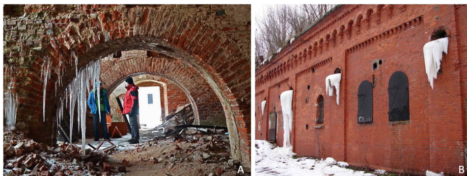
Fig. 9 Fortress buildings in winter. "Fixed" water leaks: A - from the earth-covered vaults of the Lower Bastille of the Silver Mountain Fortress Donjon (photo: G. Basiński); B - from the gargoyles on the elevation of the barracks of Fort I of the Toruń Fortress (photo: L. Narębski)
