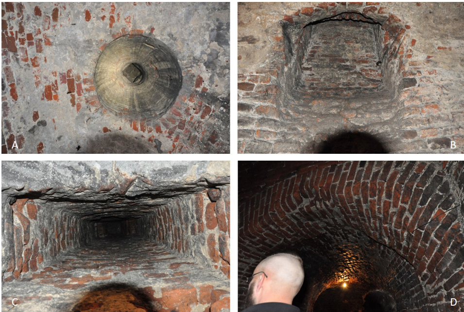
Fig. 6 Elizeum, perimeter corridor, ventilation. A - ventilation hole in the vault of the corridor, B - ventilation hole in the wall below the vault, C - ventilation duct with a blocked outlet, D - vault of the perimeter corridor 'shining' with moisture above the visitors' heads. Photo: L. Narebski, 2017
