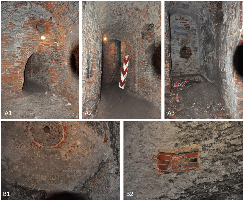
Fig. 7 Elizeum, A - perimeter corridor: lower, to the right of the contemporary entrance (A1), lower, western section, visible inlet of the ventilation shaft and entrance to the upper storey (A2), upper, view of the left wall closing the corridor (A3); B - dome: general view, visible traces of the original decor and outline of the original oculus (B1), uncovered wall fragment in the inner mantle of the dome (B2). Photo: L. Narębski, 2017
