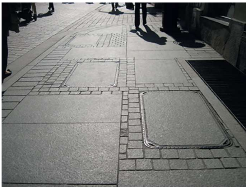
Fig. 3. The sidewalk composed of smooth stone slabs, cut paving sett and underground infrastructure manholes with smooth covers allows pedestrians to move easily across its entire width; Toruń, Poland (photo by K. Kaperczak).
