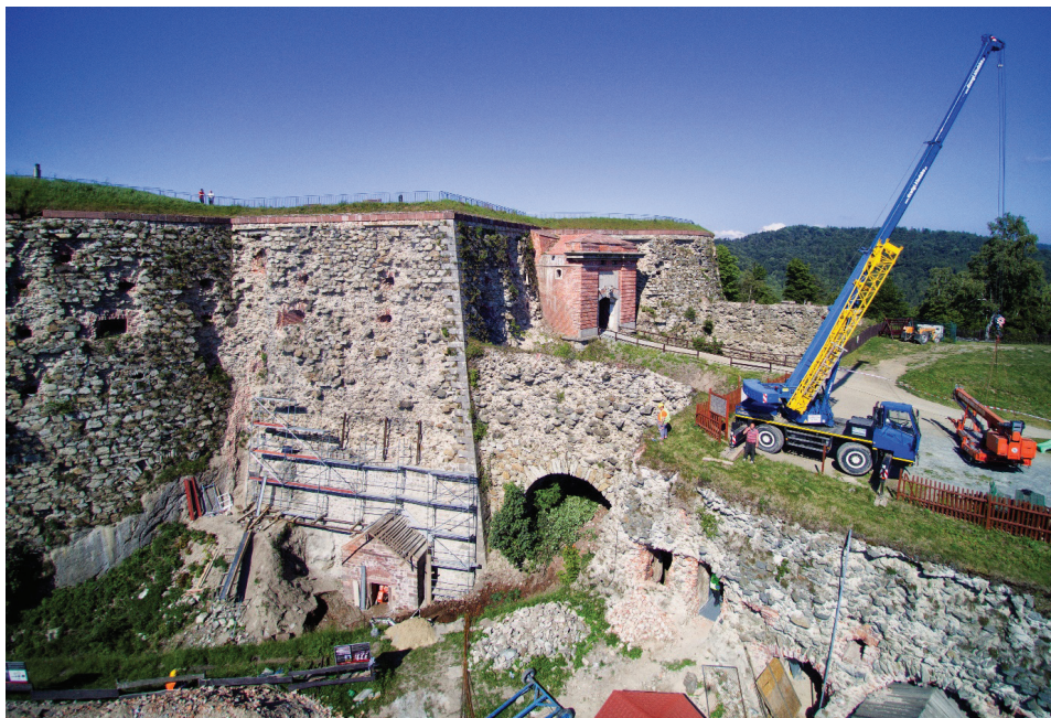
Fig.2 Renovation of the keep tower of Srebrna Góra Fortress, photo: G. Basiński
