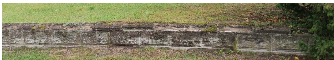
Fig. 29 Detail of the original retaining wall in the greenery area at Baths No. 1, photo by M. Lisowska, 2022.
