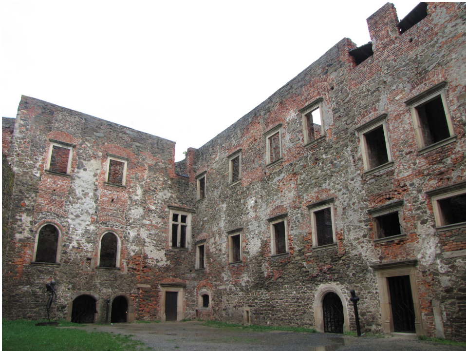
Fig. 13 Helfštýn Castle, Moravia. Castle palace before the discussed renovation, photo by the author, 2013
