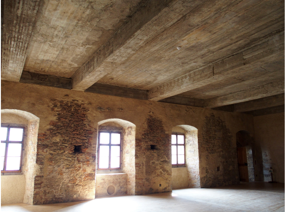
Fig. 20 Lipnice nad Sázavou Castle. A “corrective repair” from 2007–2014, photo by the author, 2019
