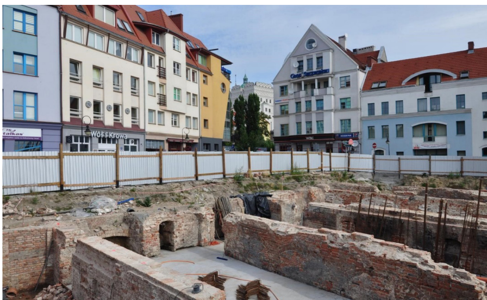
Fig. 17. Reinforcement of the foundations for the restructuring of tenant houses in Podzamcze. Photo by the author.
