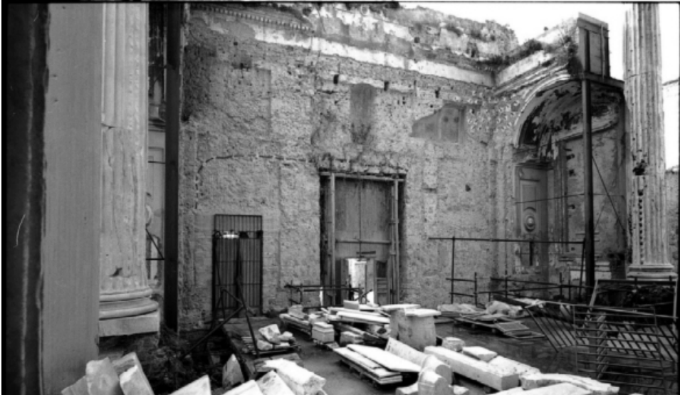
Fig. 12 Image of the original front door of the Cathedral and views of the interior of the Baroque Cathedral after the fire in 1964 and the initiation of works. [Source: Prof. L. Migliorati]
