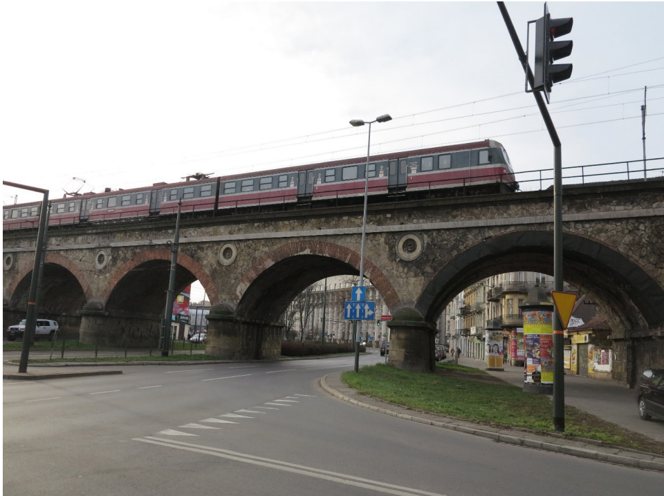
Fig. 3. Kraków, railway viaduct from 1863 before demolition and reconstruction using new technology. An example of the relativization of the approach to the monument. (by A. Siwek)
