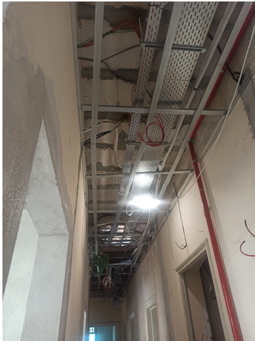
Fig. 10. Thessaloniki State Conservatoire, view of a typical, conventional first-floor ceiling, allowing concealment of equipment in a suspended ceiling. Photo: Author
