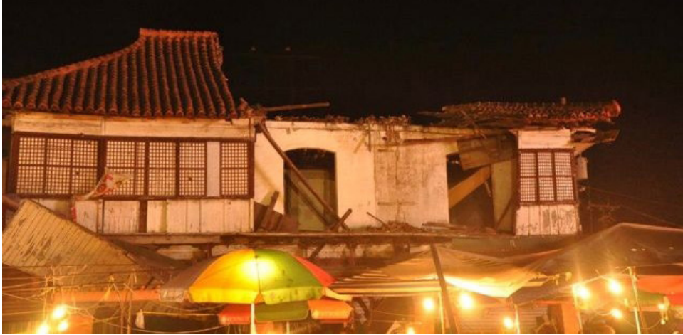
Fig. 4. The collapse of the original structure following systemic gutting of its interior components (Burningbatsu, 2012)
