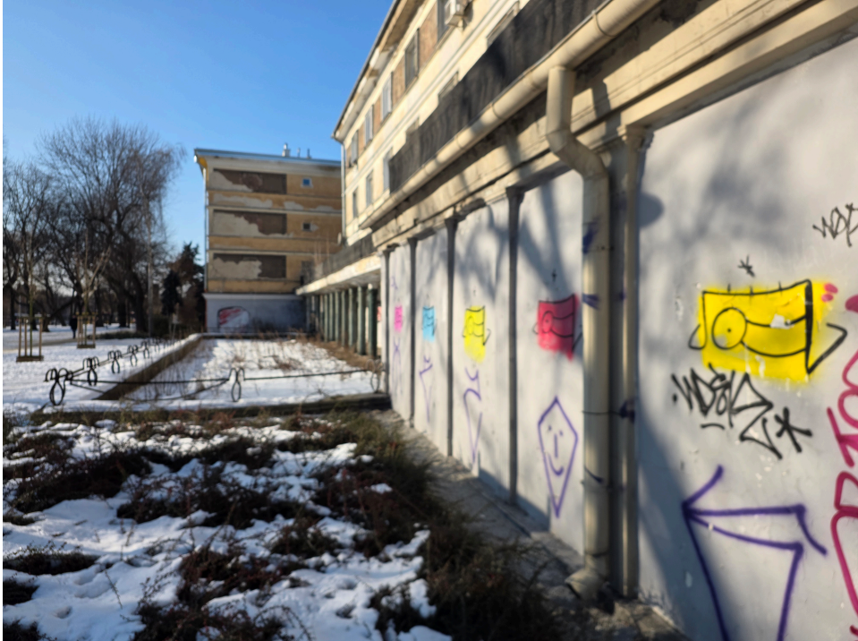
Fig. 5. Degradation of the sgraffito decorations on apartment blocks in Lodz's Old Town, photo: Ł. M. Sadowski, 2026
