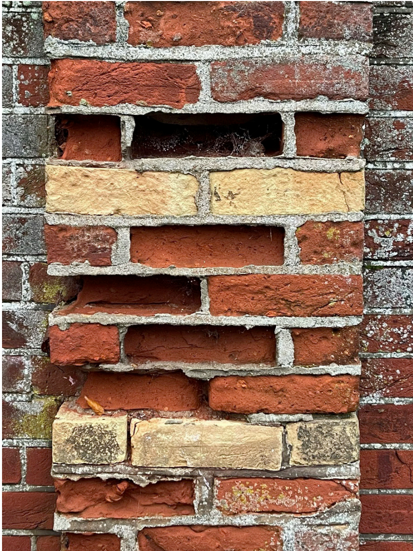
Fig. 2. Decaying brickwork, Suffolk. Photo: author
