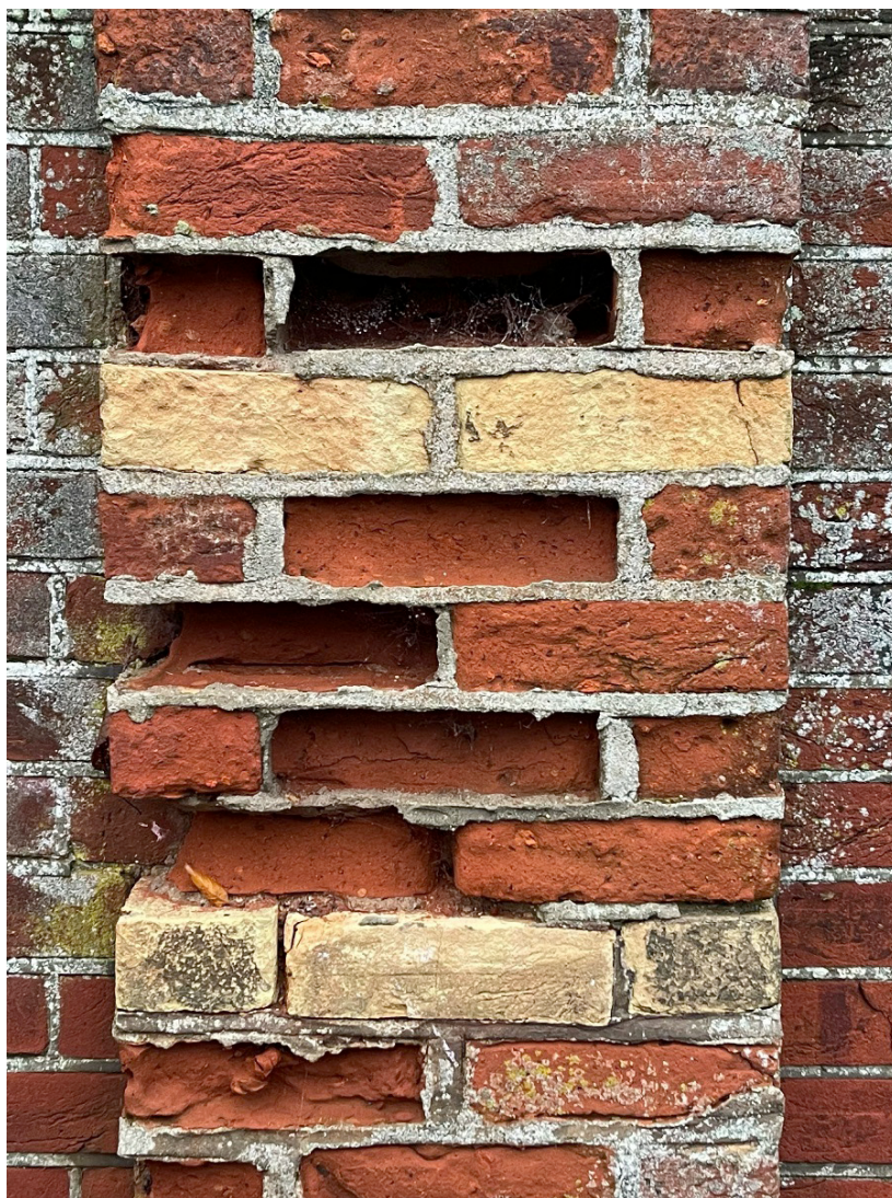
Fig. 2. Decaying brickwork, Suffolk. Photo: author
