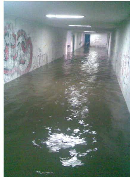
Figure 1. After intense rain water inundated the underground pedestrian passage under railway in Kostrzyn Wielkopolski in June 2010 (Kowalczak et al., 2010)
