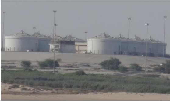
Photo 12. Mafraq sewage treatment plant. Closed sedimentation fermentation chambers (anaerobic digesters). UAE (photo by W. Sobczyk)
