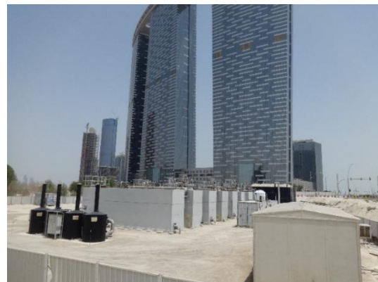
Photo 11. Modern municipal sewage treatment plant on the Reem Island. Abu Dhabi (photo by W. Sobczyk)
