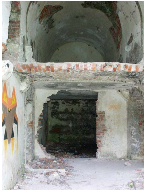
Fig. 20. Rooms No. 25 and 26. View of the entire room. Numerous loosening of plaster and cavities in bricks.
