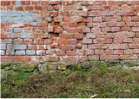
Fig. 17. The northern part of the Red Barracks. Biological corrosion of the plinth in the form of mosses and lichens. Chemical corrosion of bricks.
