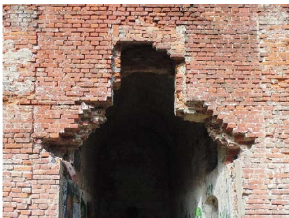
Fig. 15. The northern part of the Red Barracks. Significant shortages and cavities in the wall.
