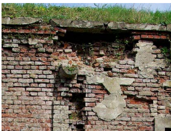
Fig. 14. The southern part of the Red Barracks. Extensive losses of bricks and stone cornice. Visible biological corrosion of a drainpipe and chemical corrosion of bricks.
