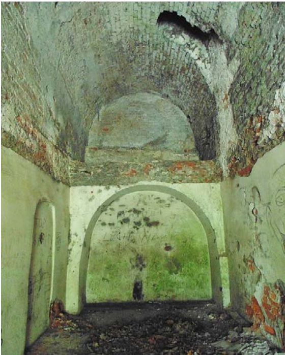
Fig. 19. Room No. 16. High degradation degree is visible. Numerous defects and cavities in the surface of walls and vaults. Strong biological corrosion and high moisture content in the back wall.
