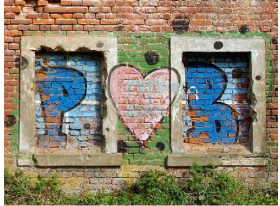
Fig. 18. The northern part of the Red Barracks. Mechanical damage to stone bands. Vandalism in the form of graffiti.
