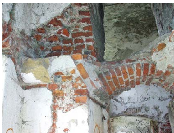
Fig. 22. Rooms No. 25 and 26. Extensive cavities and damage to bricks on the wall and door lintel.
