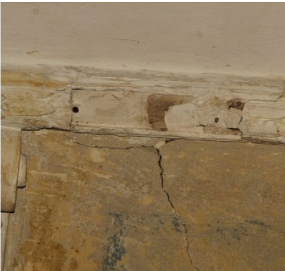
Fig. 7. Cracks on the surface of the vaults and loss of the molded ceiling decoration. Probe before the conservation, 2012. Photo by S. Hetmanchuk.
