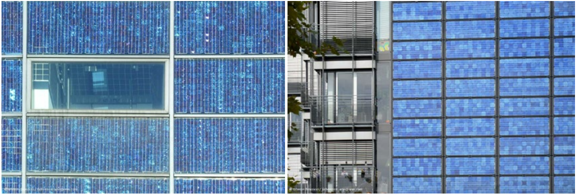
Fig. 2. Possible use of different types of cells on facades: a) monocrystalline (m-Si) cell used in the building in Punkthäuser Wilmersdorfer Straße, Freiburg (arch. Rolf + Hotz architekten, 2001, b) polycrystalline (p-Si) used in the building in SMA building nr 6, Niestetal (arch. HHS Planer+Architekten AG, 2002) – photographs by M. Muszyńska-Łanowy.
