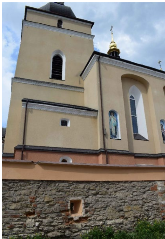
Fig. 14. Photo of the defensive wall around the Tserkva of the Nativity of the Virgin Mary in Rohatyn with a loopholes for muskets, which are arranged with an interval of 6–7 m.
