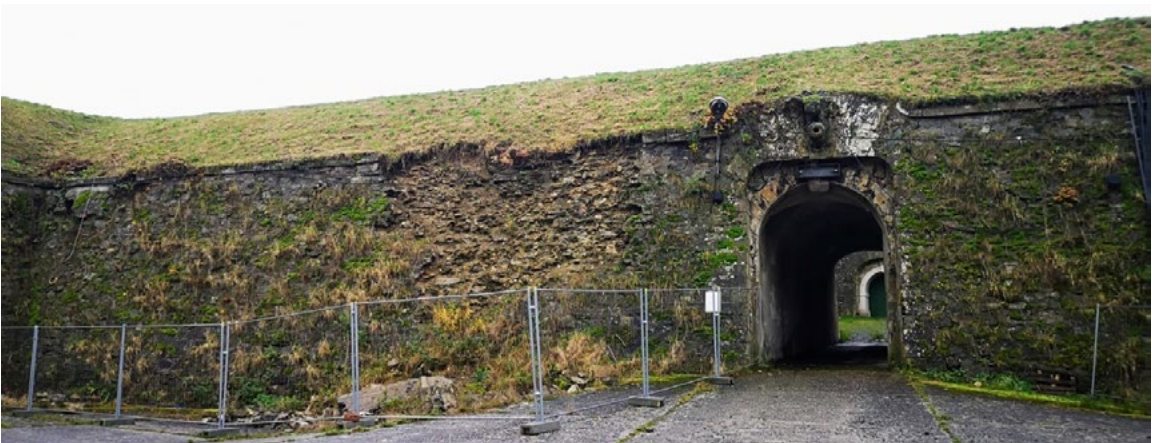
Fig. 9. Photograph showing further degradation of the wall (2020) – authors' own photograph
