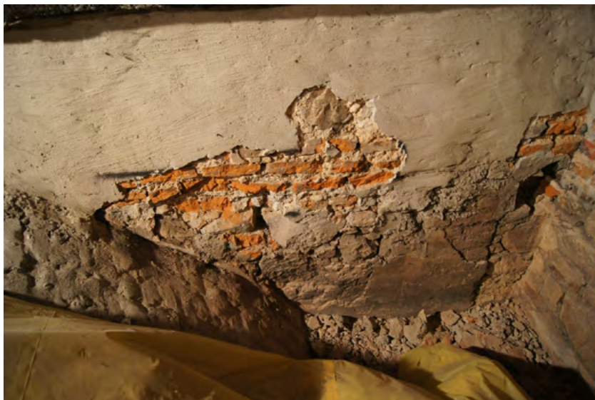
Fig. 1. View of the chancel wall from the attic over the nave with plaster relics visible, to which current vaulting was added
