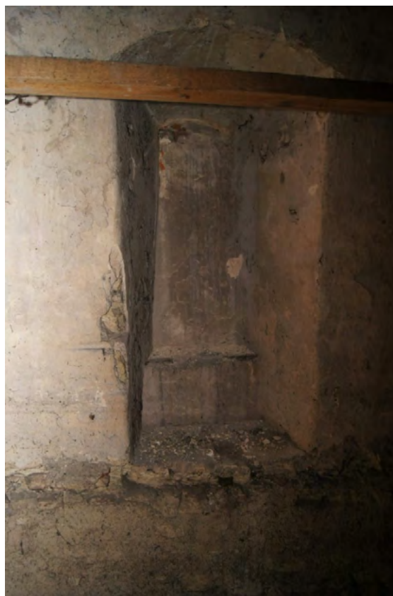
Fig. 3. Northern wall of the presbytery, view from the attic over the sacristy with the opening leading to the presbytery visible
