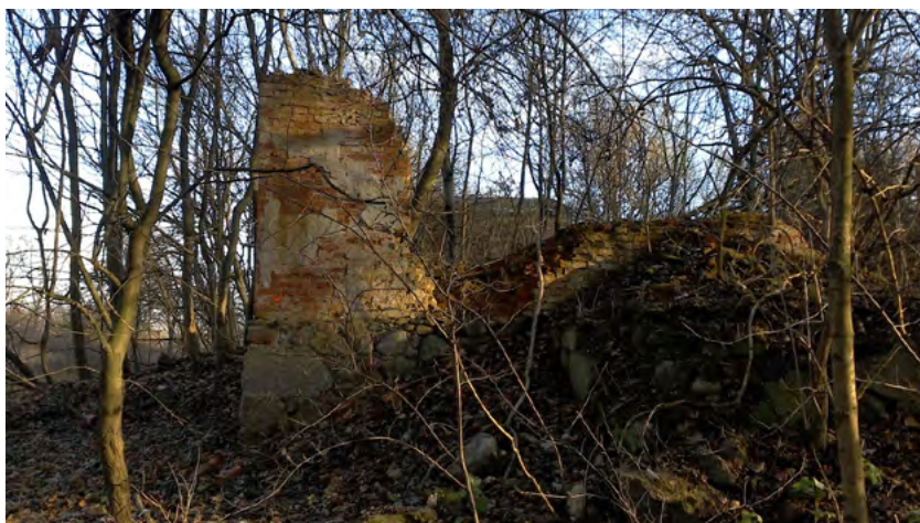
Fig. 4. Part of the elevation wall of the XIX century mansion in grórkowo, author's collection
