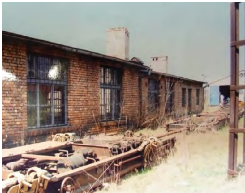
Fig. 1. One on the buildings in the Narrow-Gauge Railway in Mława, author: Wanda Gołębowska
