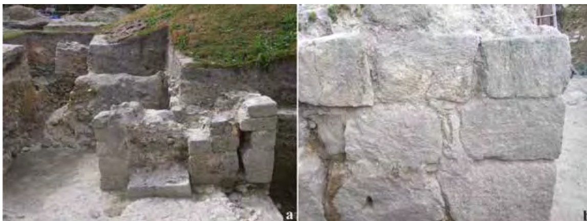
Fig. 2. Preserved elements of buildings made of glauconite: a – the entrance gate to the palace part of the castle, b – a fragment of the wall around the perimeter of the southern part, built of glauconite (photo S. Gołub)
