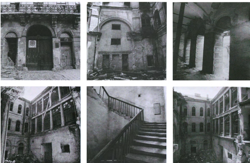
Fig. 5. The condition of the building at Mickiewicz Square 9 after the collapse of a part of the wall in 1997. Photo by I. Kostetskyi (Bevz, 2005)
