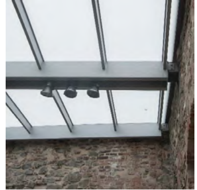
Fig. 24. Lighting mounted on roof steel beams, 2022, by K. Drobek
