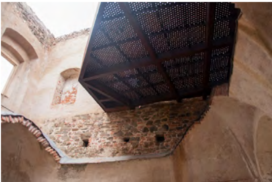
Fig. 10. Corten footbridge on the second level of the palace, glass room roofing and roof drainage, 2022, by K. Drobek
