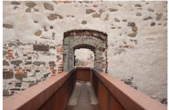
Fig. 9. Corten footbridge on the second level of the palace, 2022, by K. Drobek
