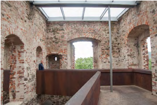
Fig. 8. Corten footbridge on the second level of the palace, glass room roofing and roof drainage, 2022, by K. Drobek
