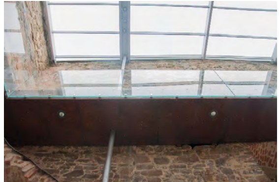
Fig. 13. Roof drainage pipe to the inside of the building, 2022, by K. Drobek
