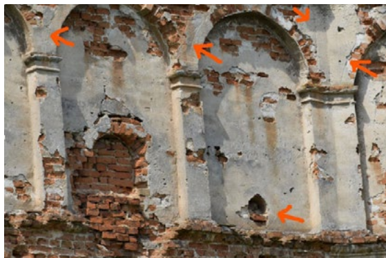
Fig. 22. The photo of the arcade belt of the upper part of the outer wall of the Stare Selo castle. Arrows indicate traces of marking for painting on plaster. Photo by M. Bevz, 2019.
