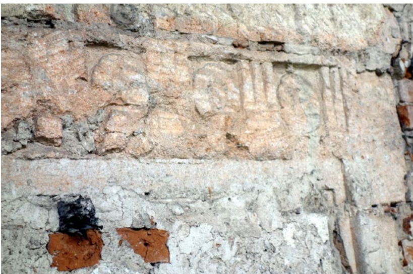
Fig. 12. Fragment of the south wall of the castle in Pomoriany. The carved window framing is made in limestone. The scenery is made up of carved rosettes and triglyphs arranged alternately. The carved forms were partially cut down during the rebuilding of the castle in the 17 th century. Photo by M. Bevz, 2017.
