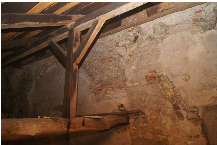
Fig. 4. Northern wall of the presbytery, view from the attic over the sacristy with the negative after two vaulting lunettes visible
