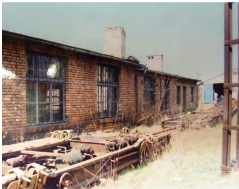
Fig. 1. One on the buildings in the Narrow-Gauge Railway in Mława, author: Wanda Gołębiowska
