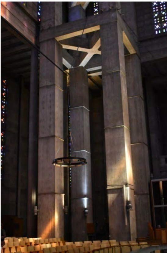
Fig. 7. Visible one of the four groups of four pillars supporting the tower. Source: Szumigala P.P.
