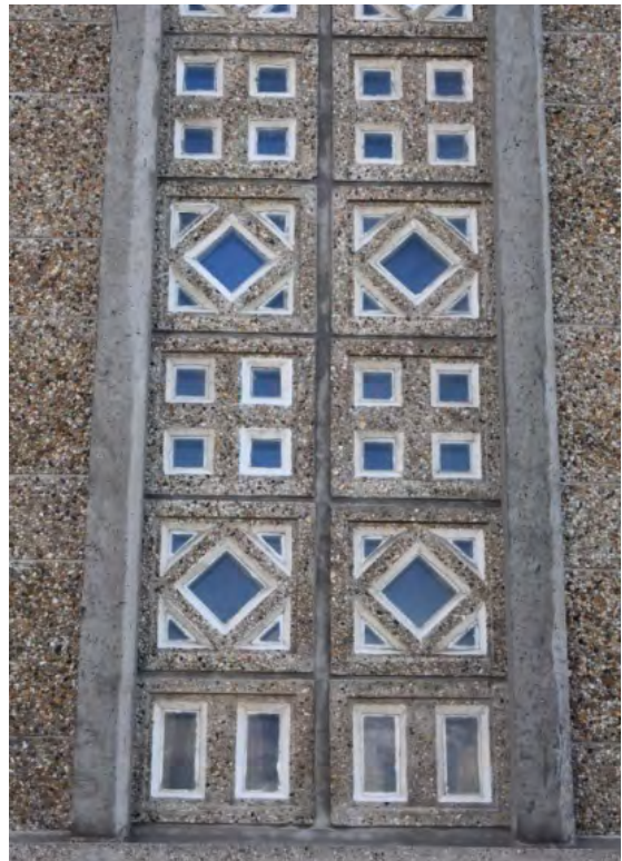
Fig. 6. Detail on the façade of the church – visible stained glass windows, concrete bands and the structure of the wall. Source: Szumigala K.O.
